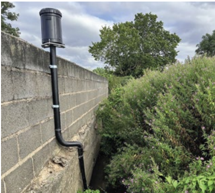
Sensors installed in the Strine IDB to monitor drainage channel and river water levels. Both sites also fitted with automatic rain gauges and telemetry for remote connectivity.
